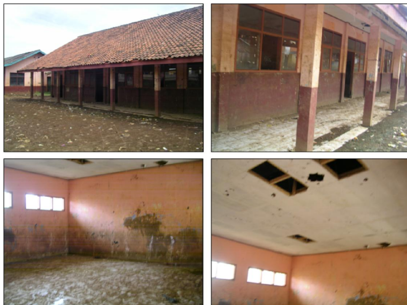
Figure 6 Elementary School Building in Cieunteung Village, Baleendah District, destroyed by flooding
